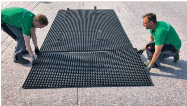
Figure 3: Installation of additional FKD 25 without Base Plate to create the spacing according to the installation plan.
